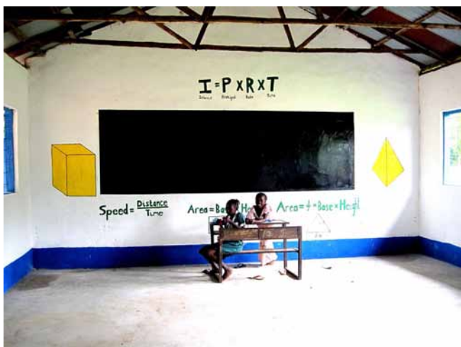
Fig. 20: A classroom block at the Lower Basic School in Gunjur (Photograph by Lilli Loveday©)
